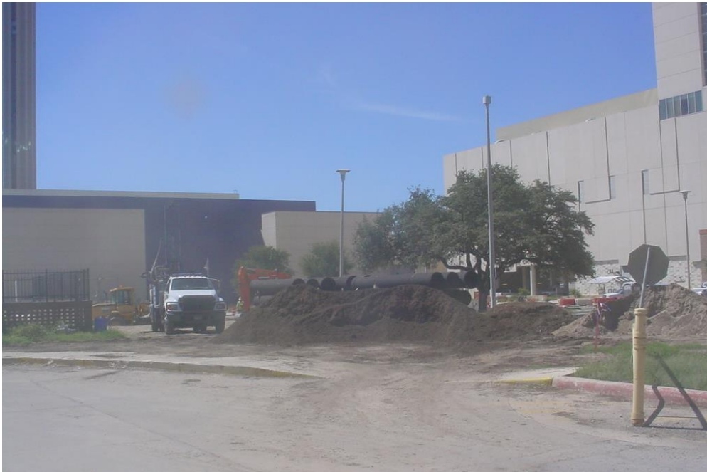
Photo 2 – View looking towards the southwest from near Boring B-3, at the drilling operations of Boring B-2.
